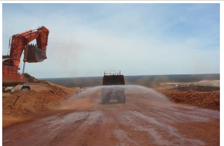
Fugitive dust can be controlled by applying water or other soil stabilizers to exposed soil surfaces daily during construction activities to avoid windblown dust.
